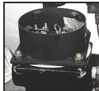
Heater mounting bolts
